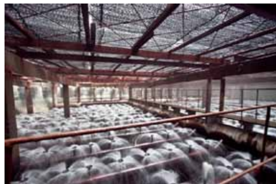
Fig. 41. The cooling system in a steam power plant (TPP-26)
