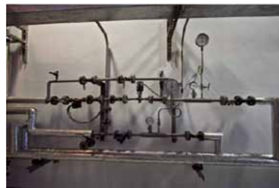
Fig. 27. Process equipment TPP-26
