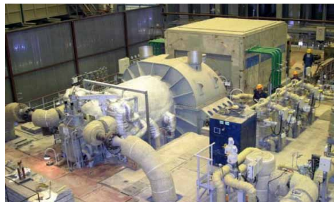
Fig. 29. CCGT-800 at Kirishskaya GRES
