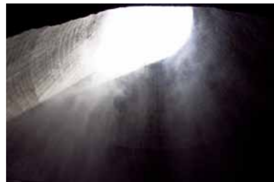
Fig. 42. The cooling tower of TPP-26
