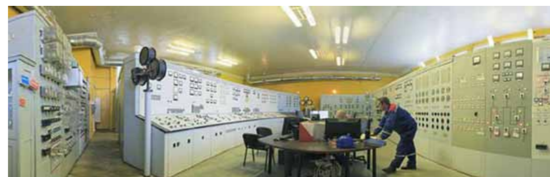
Fig. 66. Main control room at Svetogorskaya HPP
